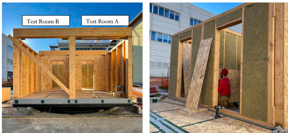
Fig. 6. Installation and assembly of the modular envelope of the BEE Lab testbed.
