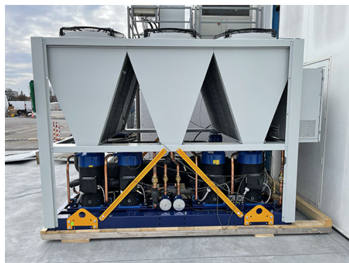
FIGURE 2. Chiller model AST 2 140 used for collecting real data.
