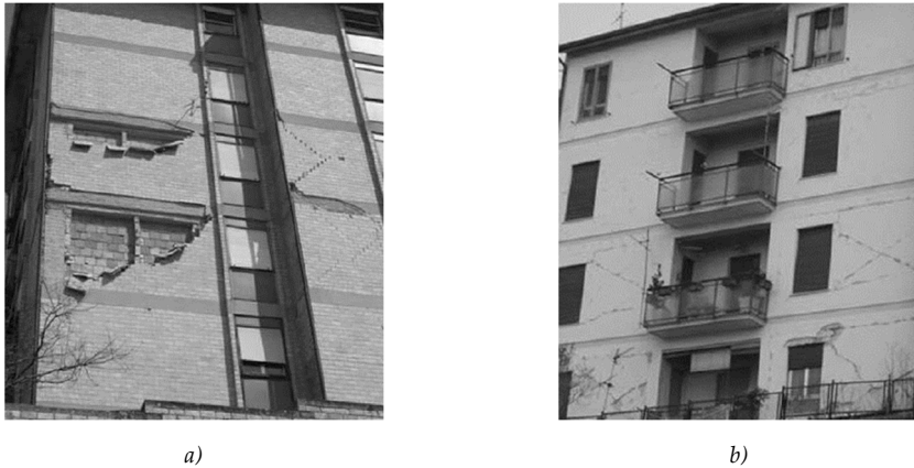
Figure 61: Infills damage on buildings in L'Aquila (IT): external leaf expulsion after diagonal in-plane cracking a) and typical X shape cracks due to reversal loading effects b) (Verderame et al., 2009c).
