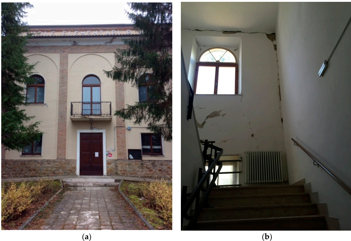
Figure 2. Gualdo, the school building after the earthquakes in 2016: (a) The entrance with the main facade; (b) Internal view with the stairway to the first floor (November/December 2016, photo IP).
