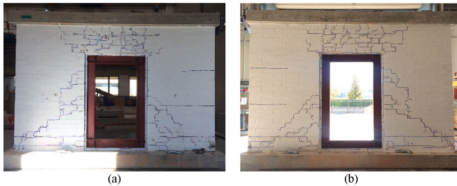
Fig. 9. Experimental crack patterns at the end of the test: front view (a); back view (b).
