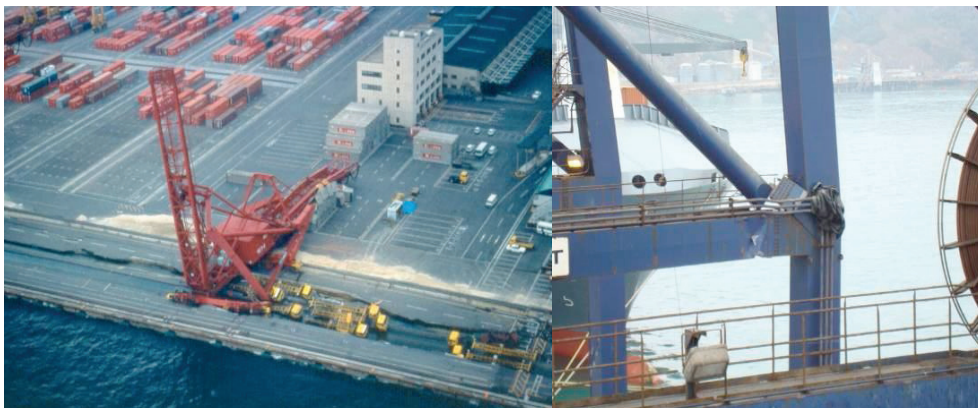
Fig. 2. Typical failure mode of cranes by earthquake.
