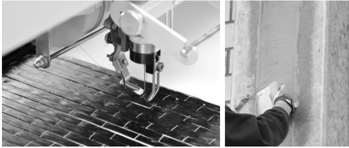
Figure 6. Production of sensor based CFRP (First: embroider of optical fiber; Second: lamination by hand at building site).
