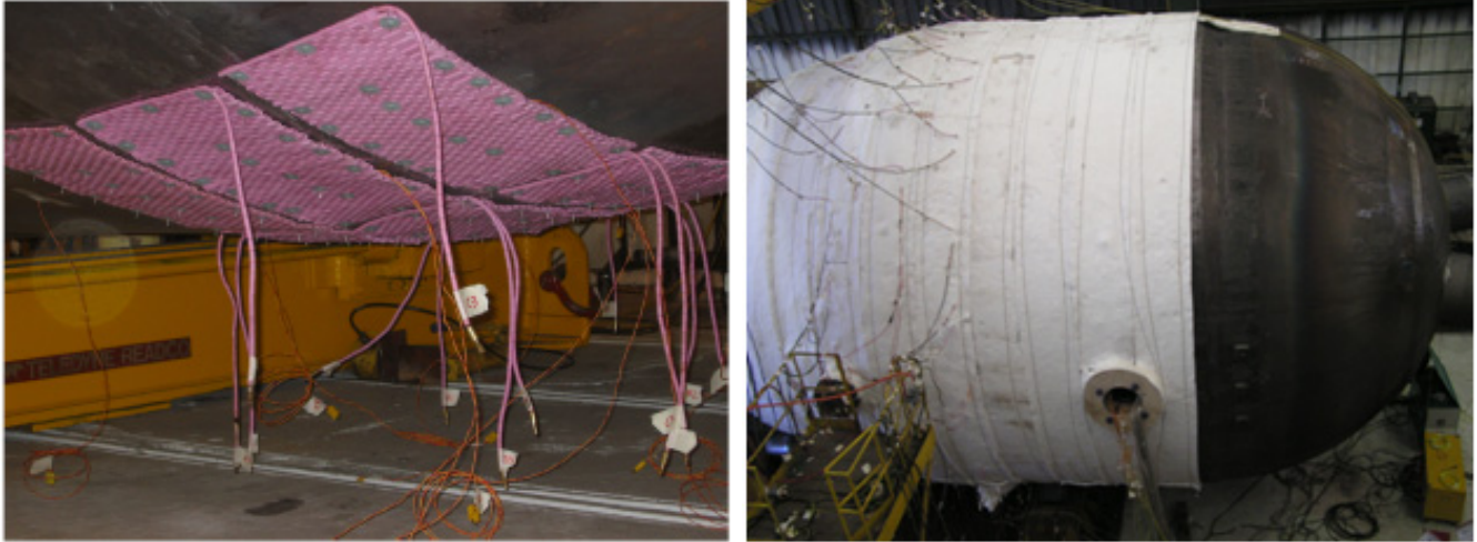
Figure 1: Heating panels attached onto the lower part of a pressure vessel in correspondence of the circumferential weld to be PWHT Treated (left); mineral insulating fibers shielding the whole zone to be heat treated (right)
