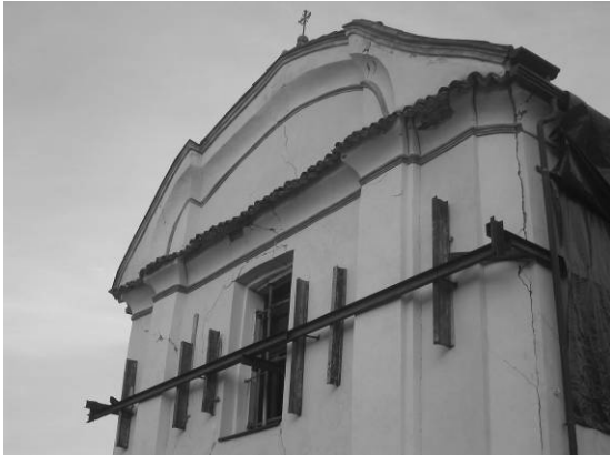
Figure 10. San Lorenzo Church (Clibbio, Brescia, Italy): external perimeter ties adopted as safety emergency provisional solution following the 2004 earthquake.
