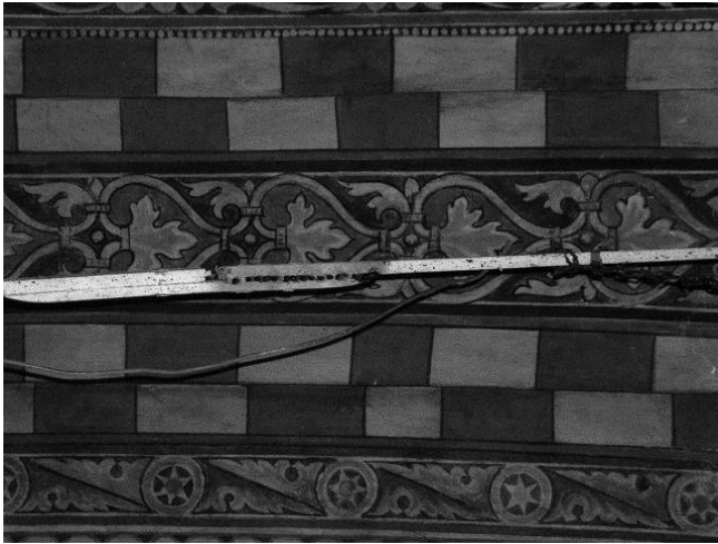
Figure 5. Detail of the welded tie rod in San Antonio Church (Manerba, Brescia, Italy). The tie rod collapsed during the 2004 earthquake.
