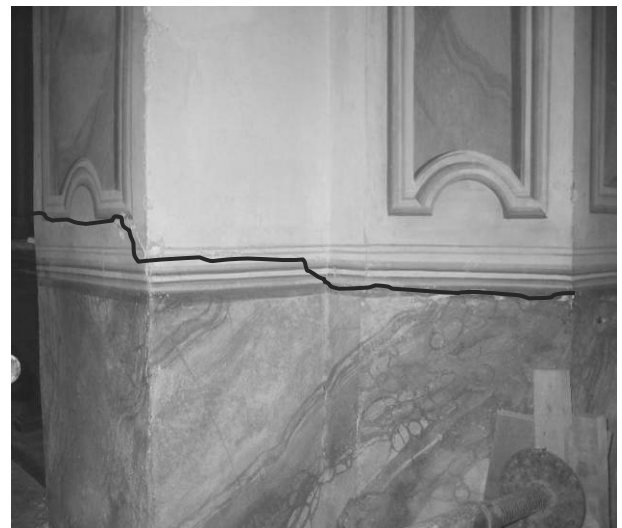
Figure 4. Detail of the horizontal crack pattern at the transverse arch abutment base induced by the seismic action.
