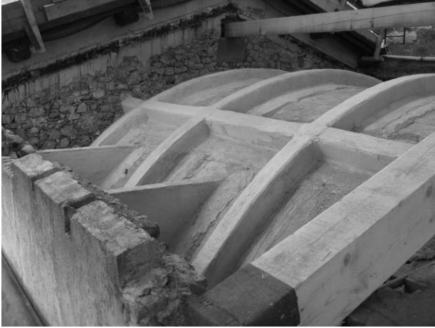
Figure 22. San Pietro Church (Roè Volciano, Brescia): light spandrel walls strengthening the single leaf masonry dome covering the presbitero.
