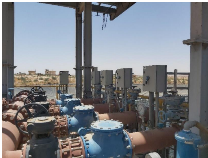
Figure A. 21 Treated wastewater pumps – Mafraq WWTW
