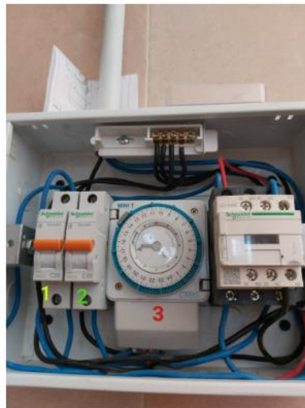
Figure F. 1 Electrical details, 1 for electricity breaker for pump 1, 2 for pump 2, 3 is the timer system
