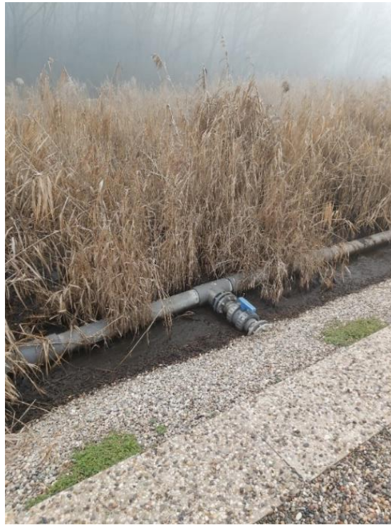
Figure A. 28 VFCWs during winter season - Carimate WWTP
