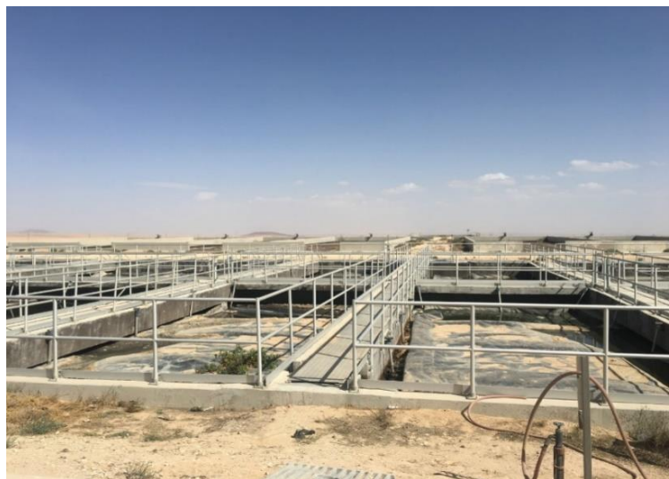
Figure A. 24 Sludge drying beds – Shoubak WWTP
