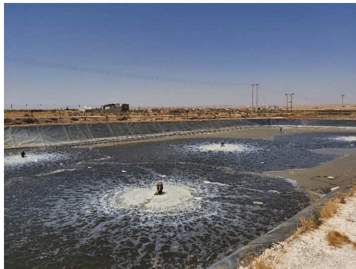
Figure A. 12 Aerated Lagoons – Mafraq WWTP
