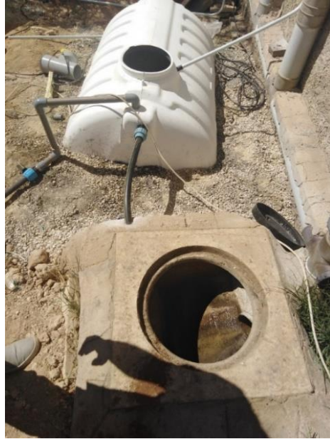
Figure G. 3 Primary settling tank – overflow to sewer system
