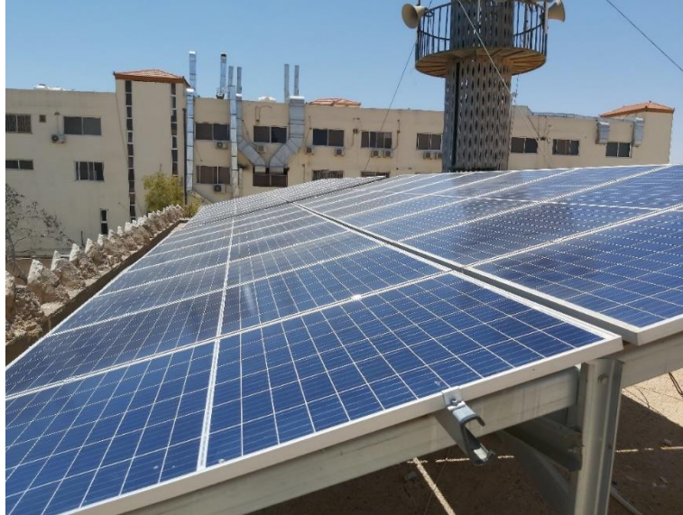
Figure 6. 4 Solar system – Roof top
