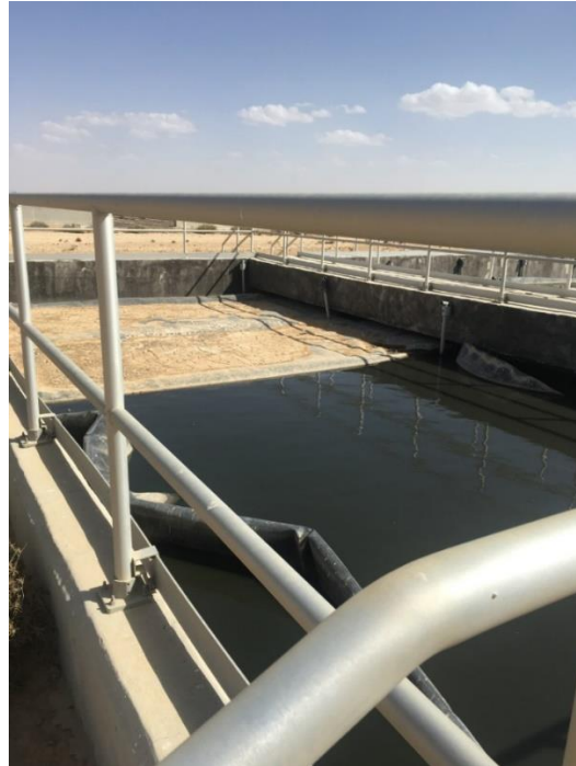
Figure A. 23 Imhoff Tank – Shoubak WWTP
