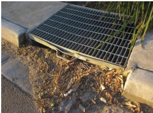
Blocked inlet – restricts flow entry, reducing proportion of flows receiving treatment.
