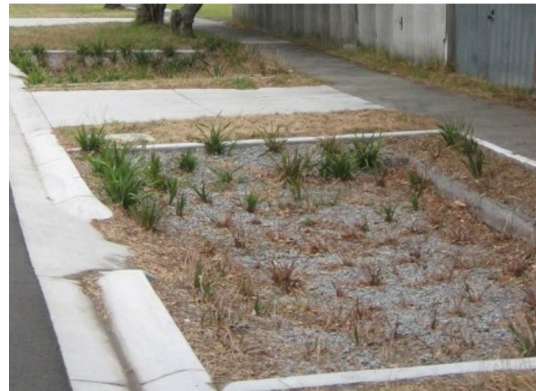
Plant die-back – severely reduces treatment efficiency and leaves media vulnerable to erosion.
