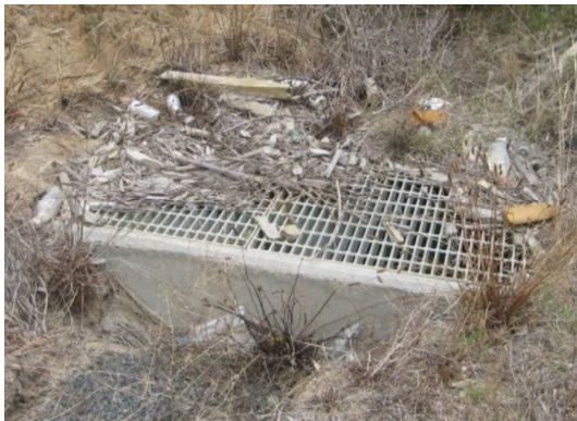
Blocked overflow grate – lead to flooding and damage to the filter and vegetation.
