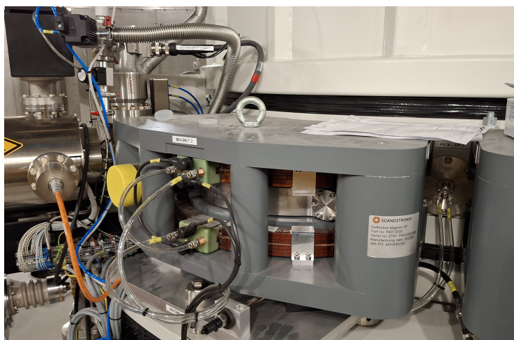
Figure 2.5: Rhodotron bending magnet (one out of nine) during the installation at Copan sterilization plant.
