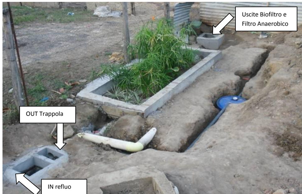
Fig. 4.36: Impianti in Venezuela
