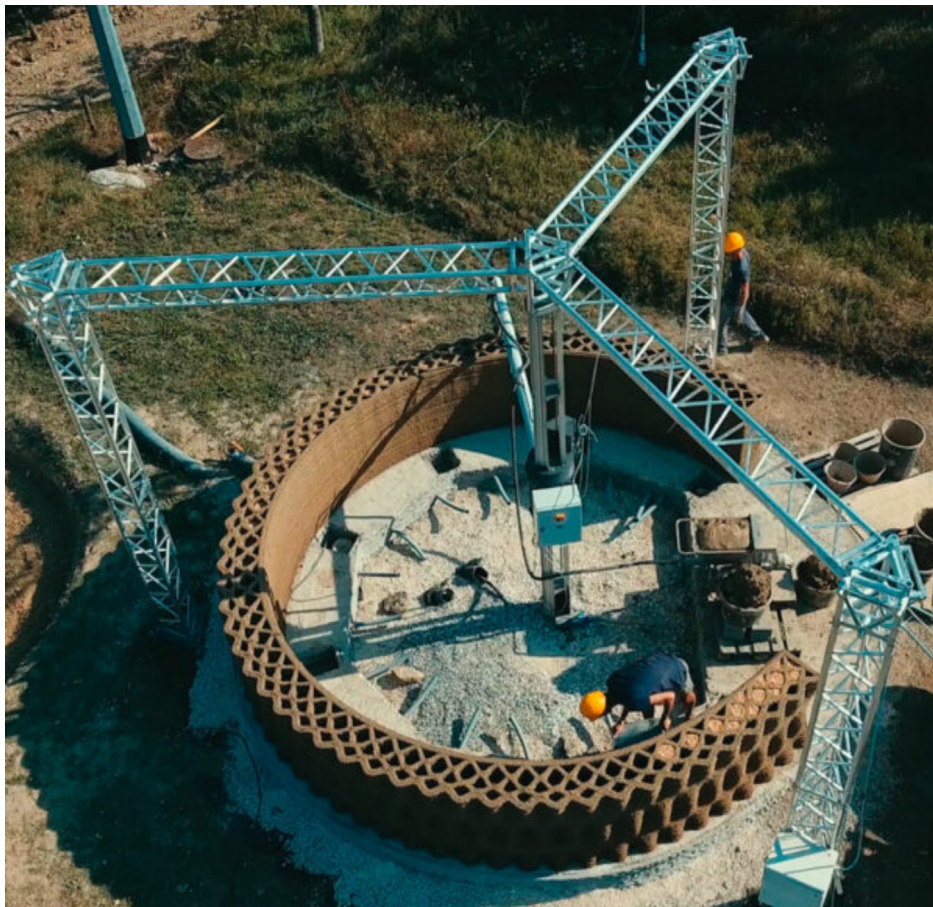
FIGURE 9: Gaia Project by Ricehouse, 3D printed house with biomass insulation built with a 3D Crane WASP printer and natural materials from the landscape nearby, in a blend of natural materials including clay, ground sand, rice straw and rice husk (Source: https://www.ricehouse.it/storie/gaia/ ).
