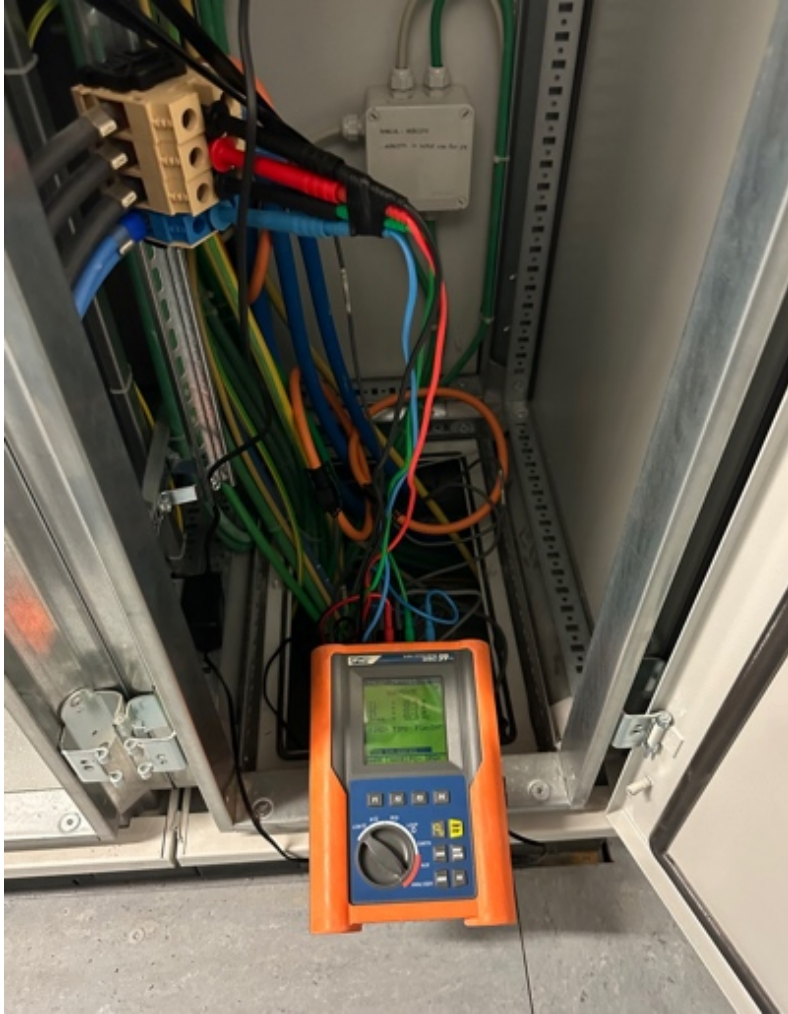
Figure 5: Measurement setup for on-site energy monitoring. Power consumption was measured non-invasively with a power quality analyser (GSC59, HT Instruments) connected to the incoming power line of the MRI electrical cabinet. The analyser continuously measured voltage, current and power parameters during routine scanner operation, allowing real-time assessment of energy demand without interfering with clinical workflow.
