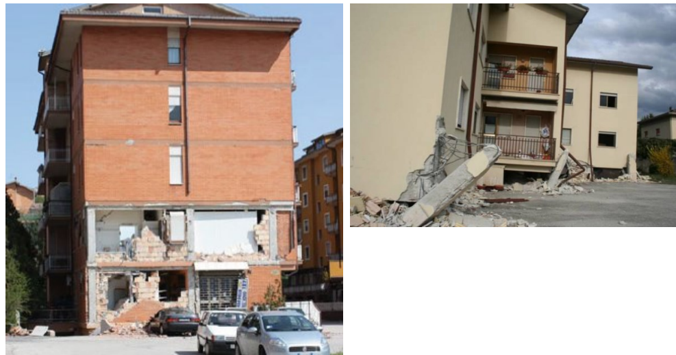
Figure 1.1: Example of collapse of infills at low storeys [1] a) and soft-storey mechanisms [4] b) after the 2009 L'Aquila earthquake.
