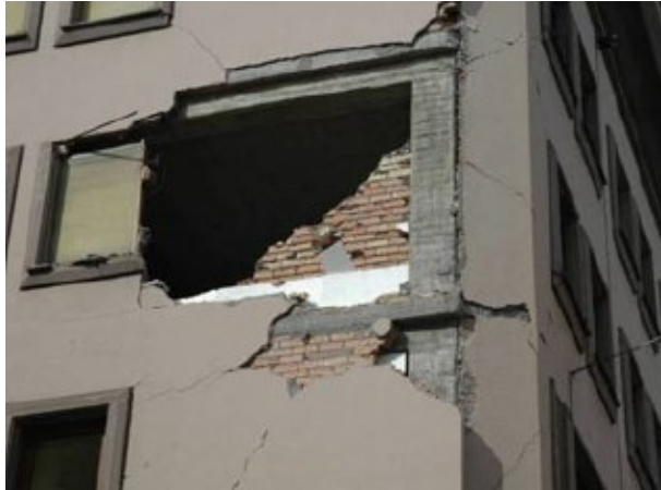
Figure 1.2: Example of out-of-plane collapse of infills at upper levels after the 2009 L'Aquila earthquake [1].
