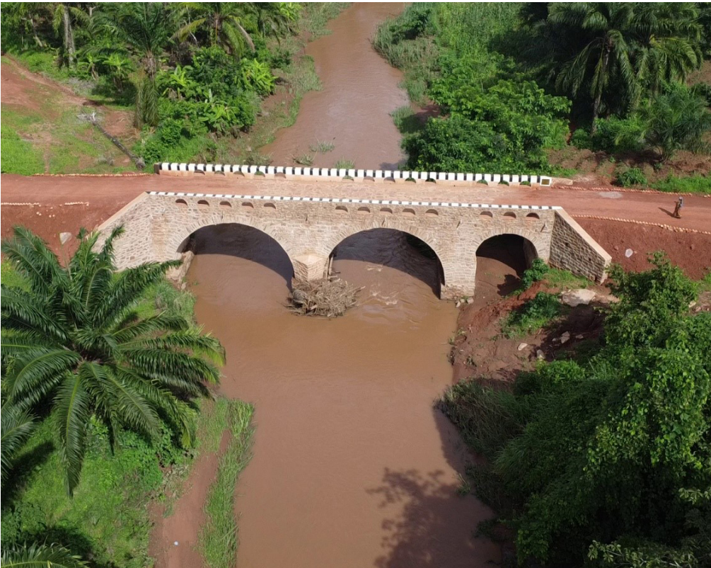
> Chankabwimba bridge creates a shortcut for villagers to reach public services and a safe alternative for the existing bridge on the main road which is in bad condition and is often submerged during floods. (25m span, 39 000 EUR) © Enabel
