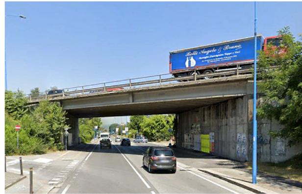
Fig. 1 – The case study bridge on the south ring road in the city of Brescia (Lombardy Region, Italy).
