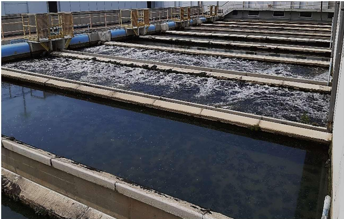
Figure 4. 19 Filtration tanks – Source SMAT S.p.A
