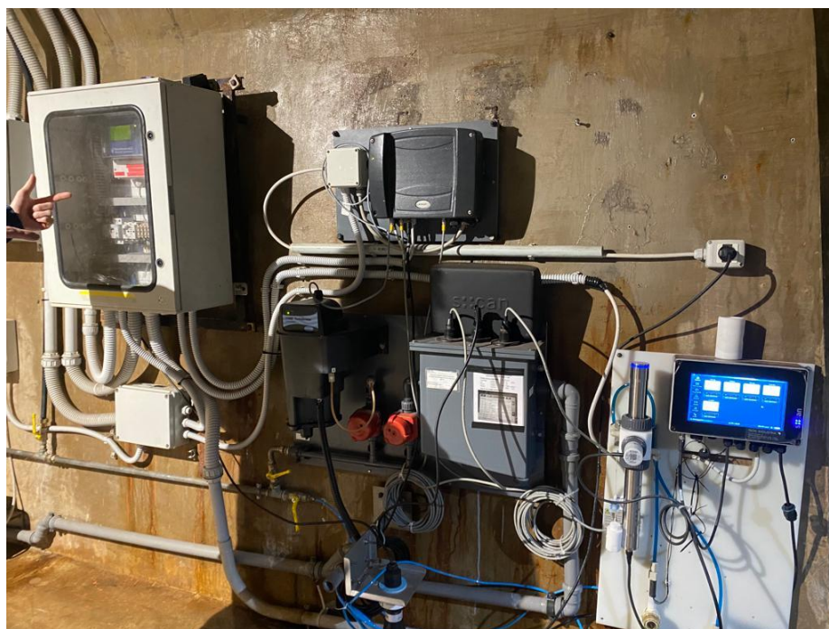
Figure 5. 29 Monitoring system installed at the Mompiano source
