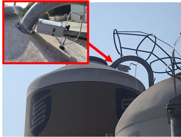
Figure 2.7 – Image of the prototype installed outside the circular fiberglass silo.
