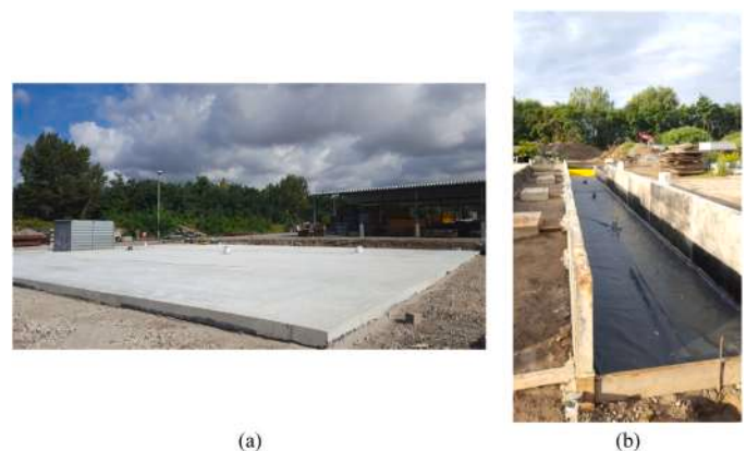
Fig. 1. Square slab after casting (a) and double plastic sheet layer of unidimensional slab before casting (b).
